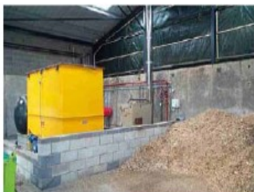
Figure 2. A Veto (80kW) wood chip boiler heating a farmhouse, two cottages, a café and business units
