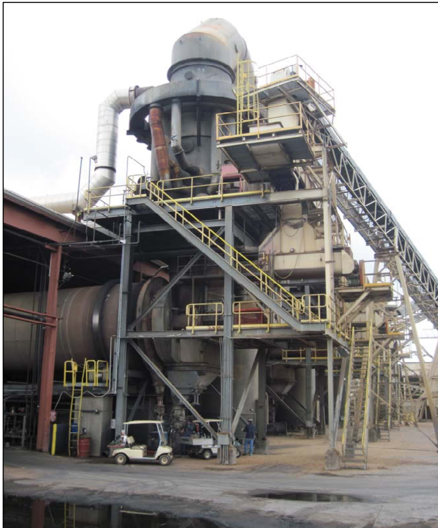
Rotary kiln, oxidizer tower, and fuel feed system
