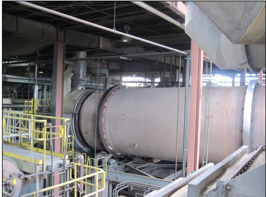
One of three rotary kiln gasifiers at Norbord
