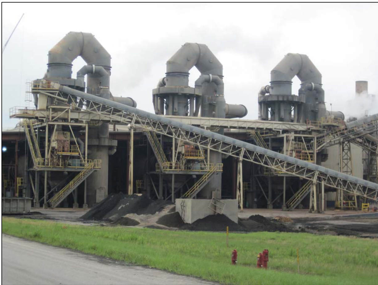
Callidus system at Norbord mill in Kinards, South Carolina – Picture shows the three vertical thermal oxidizers at each rotary kiln and the wood fuel feed conveyors.
